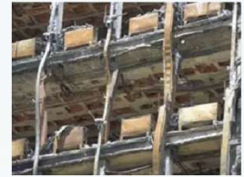
Buckling at floor 9
